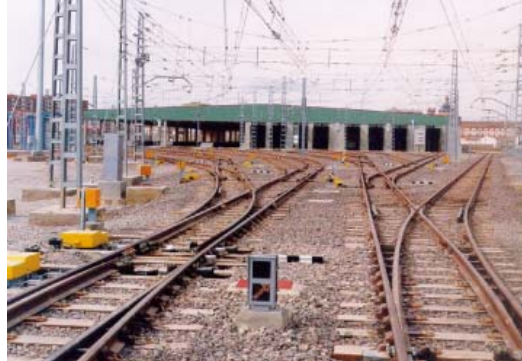
Fig. 2 –Switches and signage.
